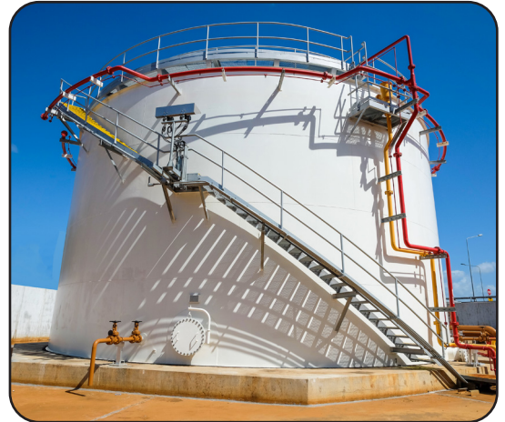
Above: An example of a container tank at an oil refinery. These tanks contained industrial mixers that would agitate the slurry contained within, with a new monitoring and alert system required to advise of the slurry status.
